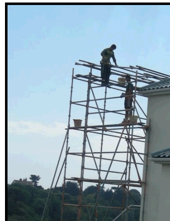
Unsafe scaffold erection in progress
