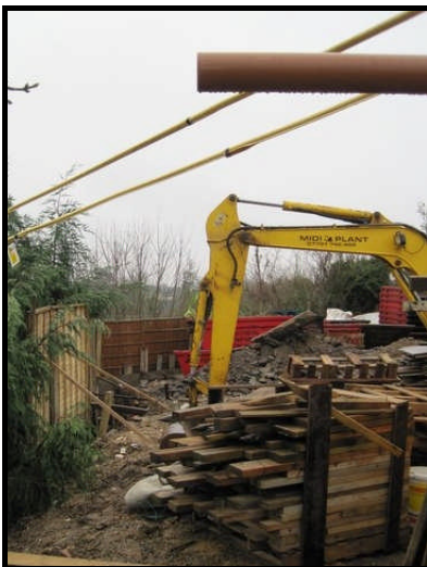
Work was stopped because of the proximity of the overhead electrical cables
