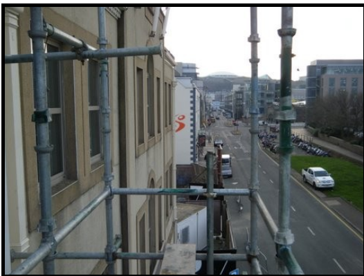
Area from which the scaffold tube fell
