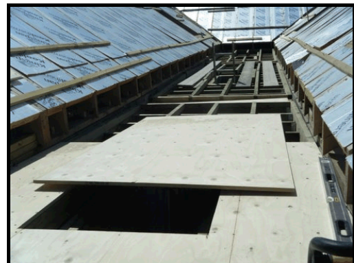
Roof area showing board removed to reveal opening through which he fell
